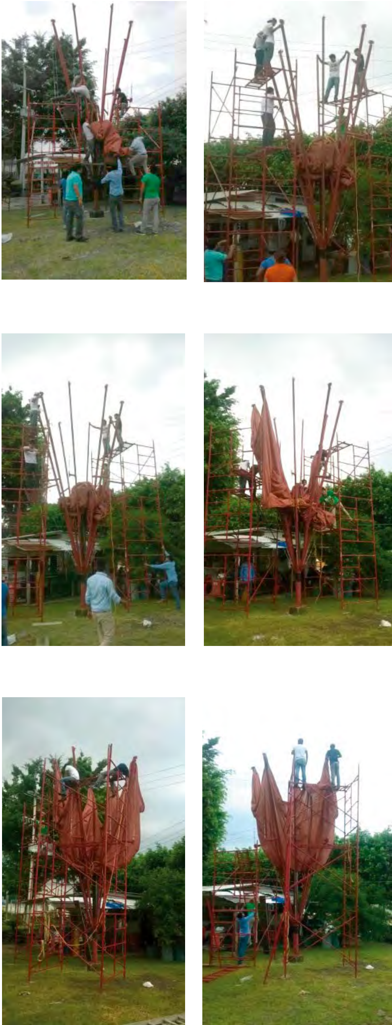
Figure 67 to 72. Subsequently, the pre-stressed membrane of the umbrella was placed, with the help of two reinforced scaffolds of 9 m. In each connection, a regulator and a 1/4" shackle were placed, which served as a flexible articulation at the time of deployment. Source: Morales-Guzmán (2013)..
