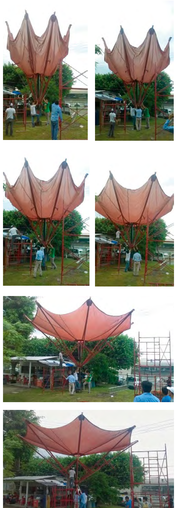
Figures 73 to 78. First deployment of the folding umbrella with membrane; this first attempt failed because regulators were half-open and this prevented the membrane from being completely tensioned. Source: Morales-Guzmán (2013).
